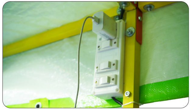
Phone Charging Socket and Switch
